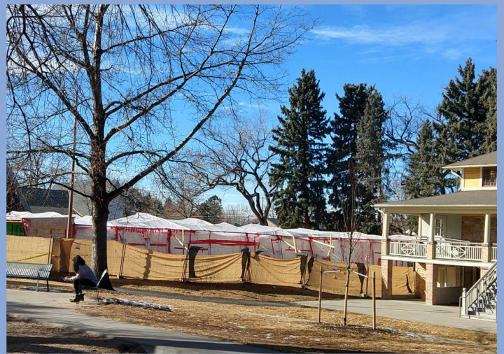
Upon completion of asbestos mitigation, Montclair Park's tennis court will be replaced with a brand new court, fence, landscaping, ADA accessible parking spaces, and improved picnic area access.
